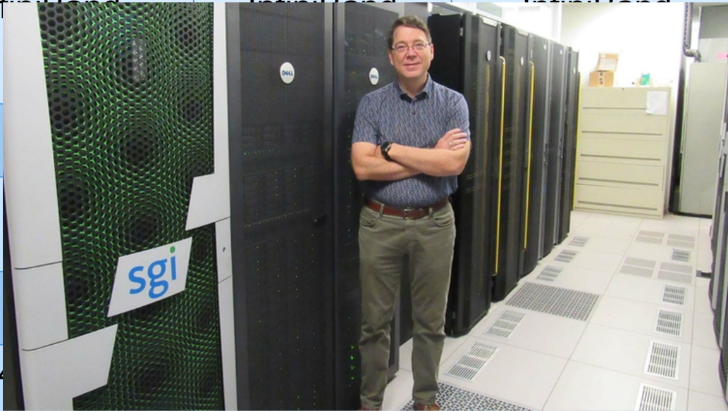
Wheeler 2400 cores in 306 nodes, 12 racks Estimated 25 Terra Floating Point Operations/second (Tflops)
